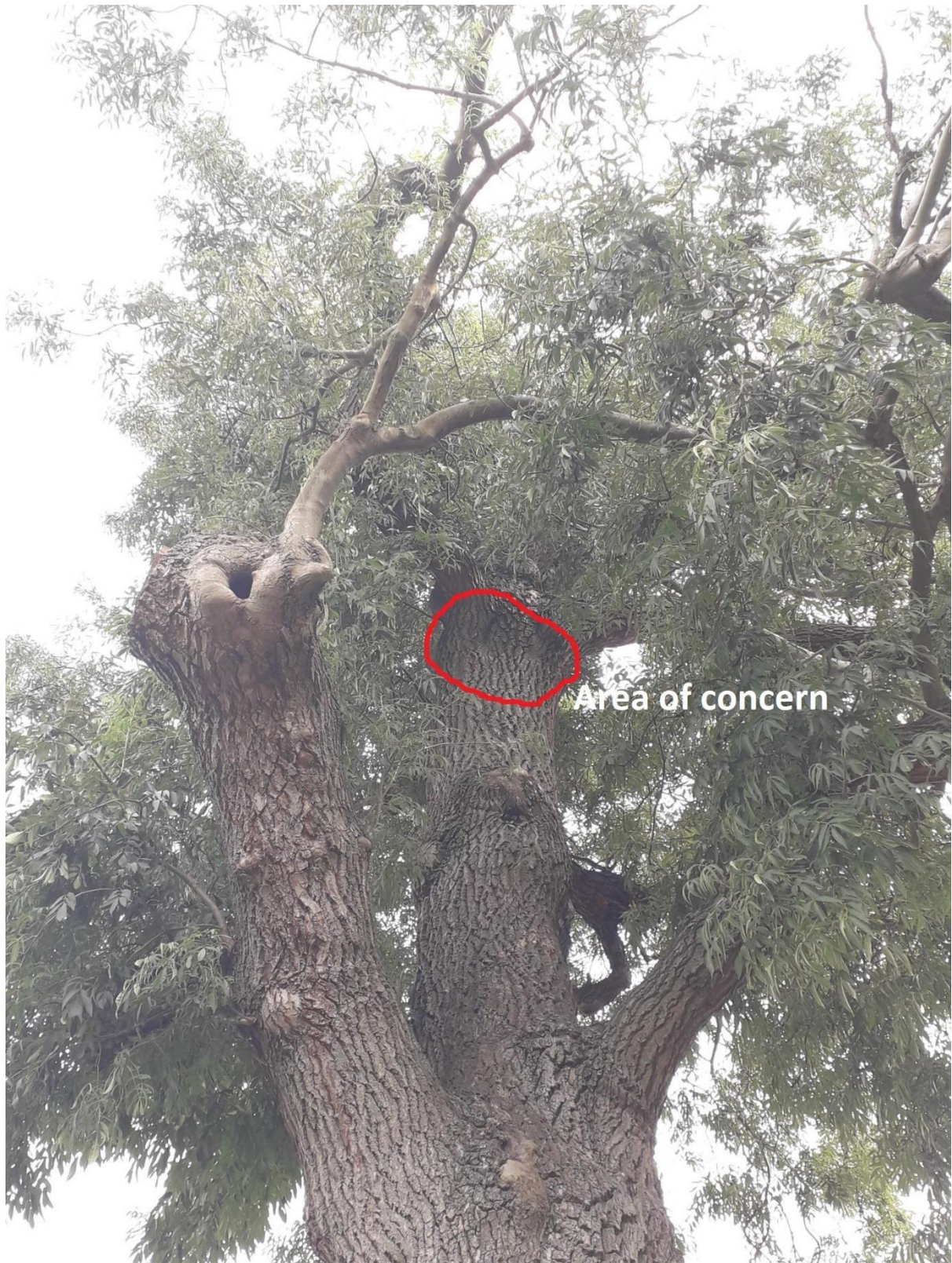
Photo 14 – areas of concern. Upper trunk. Drilling 1 to 6.
